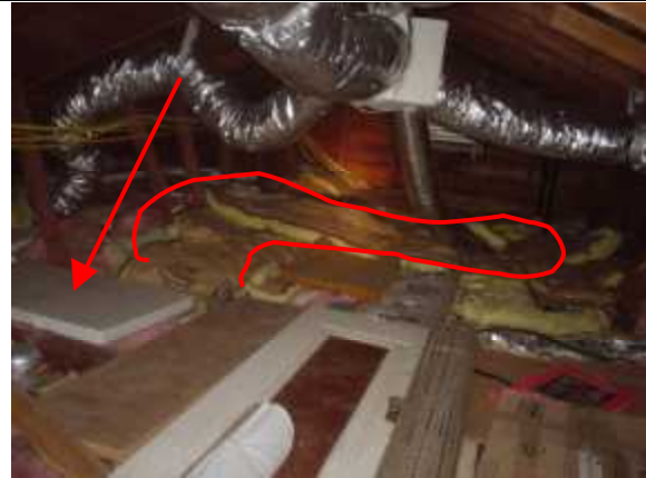
4. Insulation batts upside down; Styrofoam in attic
