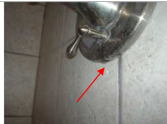
1. Leak at shower diverter
