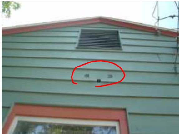
5. Exposed cladding and wire at rear
