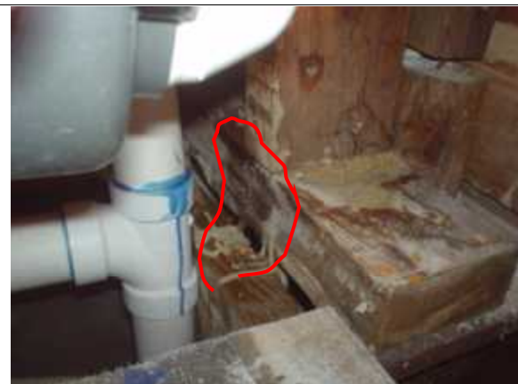
2. Water below tub from shower diverter leak
