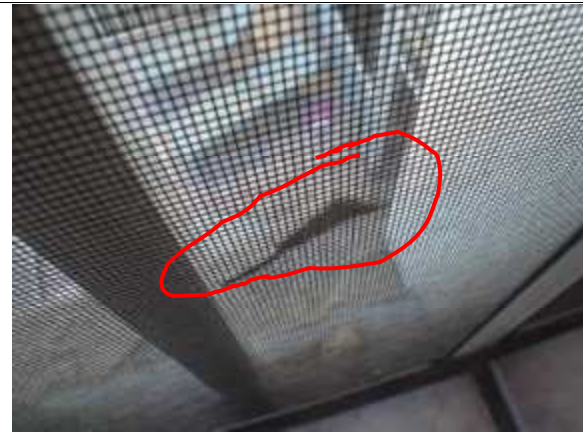
4. Loose & exposed stucco at right side of terrace
