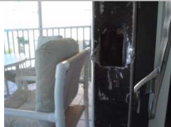
3. Damaged sliding glass door lock
