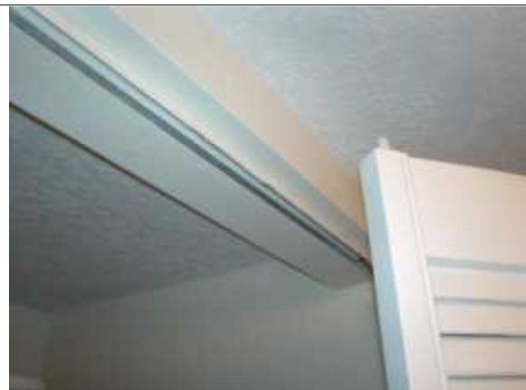
2. Laundry bi-fold door loose at overhead track
