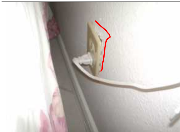
1. Loose outlet at front sleeping room
