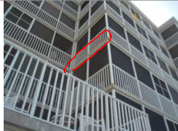
6. View from pool deck, damaged stucco
