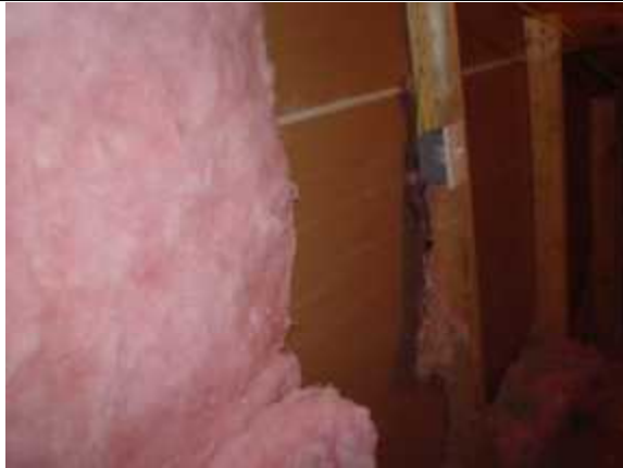
3. Missing wall insulation, stairwell
