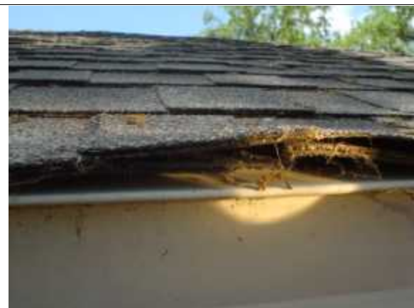
2. Raised shingles, left rear
