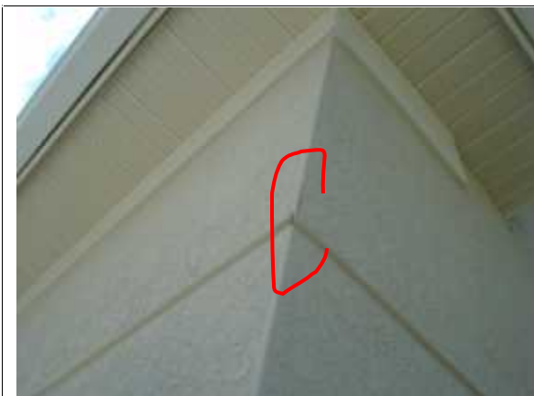
1. Typical hairline cracks in stucco
