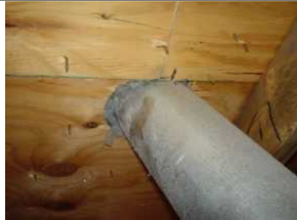
4. Clogged dryer vent
